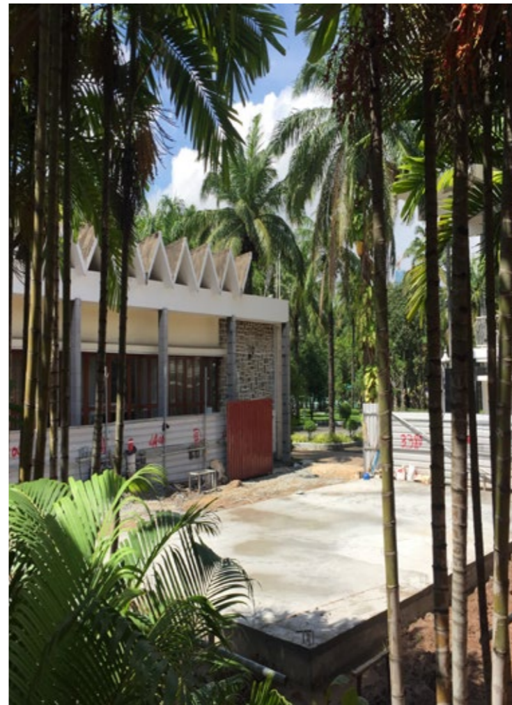
The strip footing supports a concrete slab and a stable steel structure.
